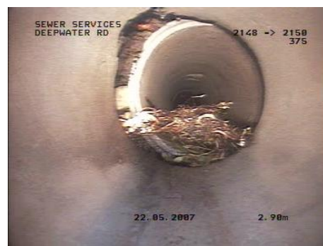
Large Displaced Joint
