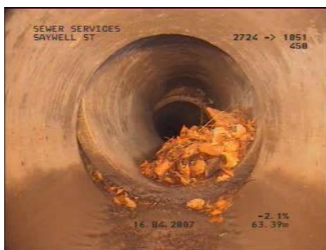
Large Displaced Joint
