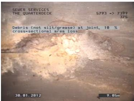
Broken/ damaged joint Minor
