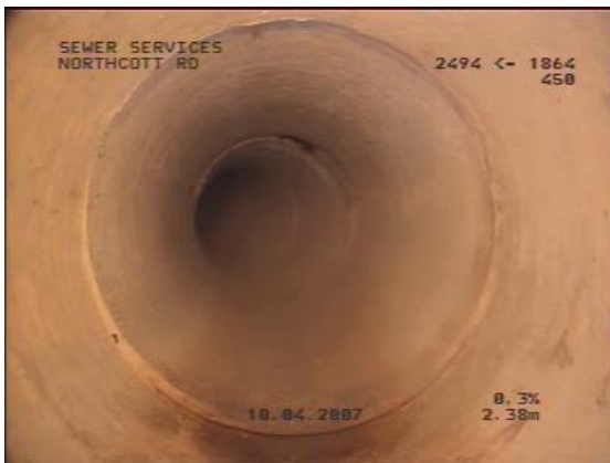
Slightly Displaced Joint
