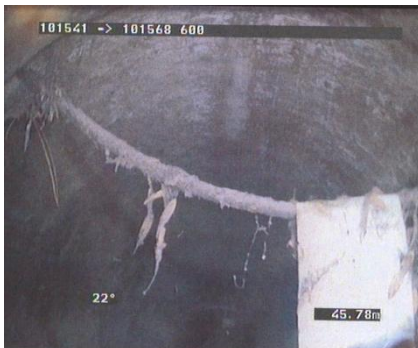
Large Rubber ring joint failure
