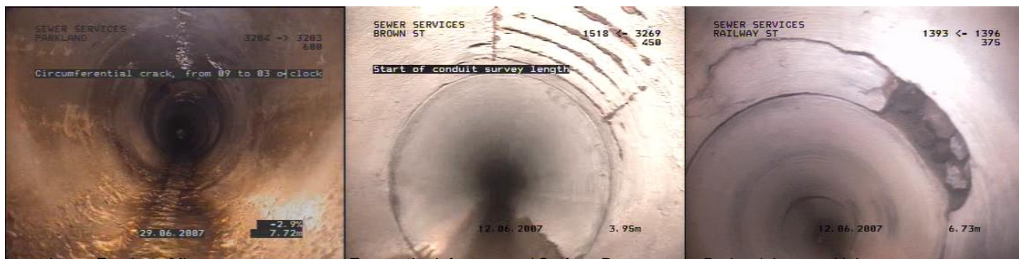
Invert Erosion - Minor
