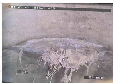
Minor rubber ring joint failure Service not affecting flow
