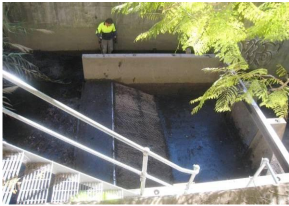
Baramy at Eastern Valley Way being cleaned.
