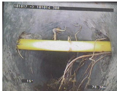
Utility Service in conduit
