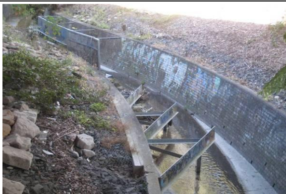
Baramy at Grandview St prior to being cleaned.
