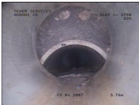
Extreme displaced joint
