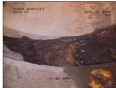
Large open joint
