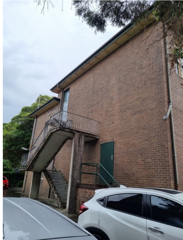
Figure 39 southern elevation of the 1932 main school building showing few openings and external fire egress stair.
