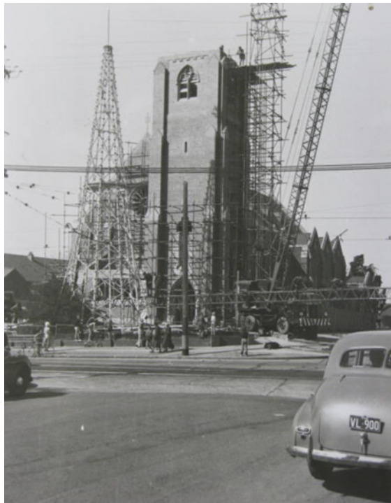
Figure 12 Spire under construction, St Leonards Catholic Church, Willoughby Road and Donnelly Road, Naremburn, 1955 (Source: Willoughby City Library, record no. 220194).
