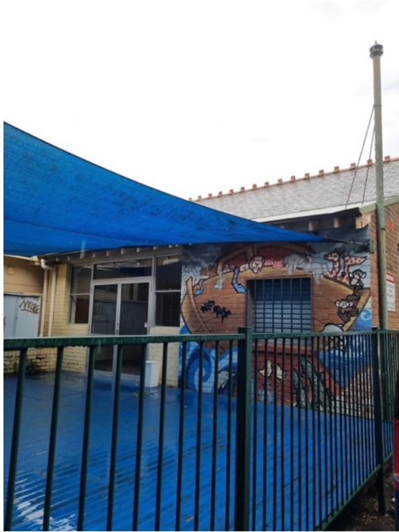
Figure 42 western elevation of the 1936 classroom building. Mural on brickwork and some openings altered/added.
