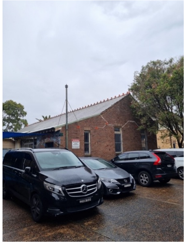
Figure 43 Southern elevation of single storey 1936 classroom building. Slate roof and decorative ridge capping likely salvaged.
