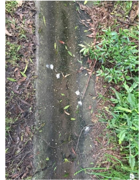
White wash in drain in front of grandstand
