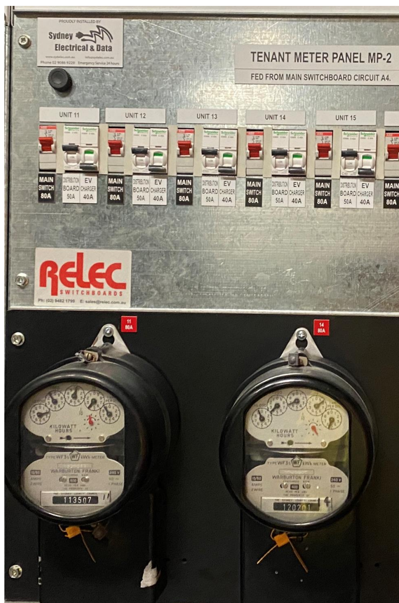
Meter Panel with 40A Sub-Mains to parking spaces for EV Charging
