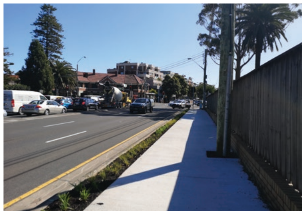
Work underway on a new shared path between Chatswood to St Leonards
