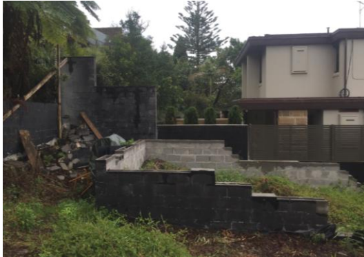
Unauthorised retaining walls in rear yard
