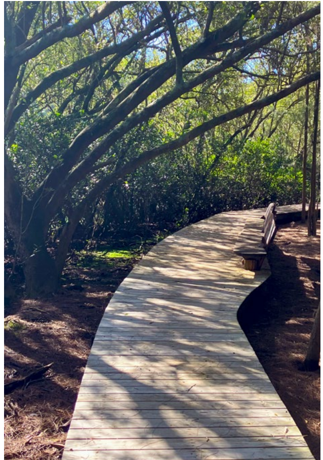
The work on the boardwalks creates opportunities for better access to the river foreshores.
